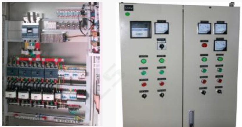
Image 3-20 Three-phase power cabinet
