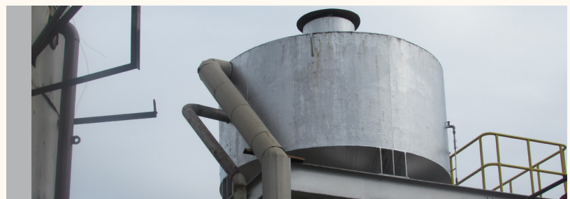
Open Vessel called a Flash Tank which releases Trapped Air Bubbles
