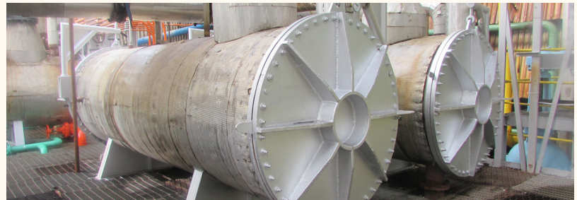
Pressurized Juice Heaters which raise temperature of cane juice to 280° Fahrenheit
