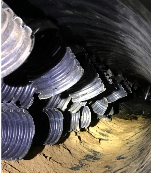
Figure 11: Installed baffles in Gray House system
