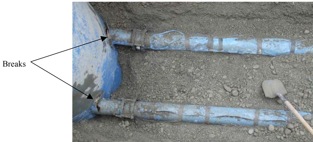
Photograph 16: Wigram Pump Station, Christchurch (PS101): Both 150mm diameter discharge pipes to the valve chamber fractured in the fibreglass pipe spool at the pump station wall.
