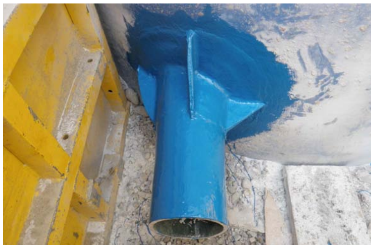
Photograph 17: Wigram Pump Station, Christchurch (PS101): Strengthened and gusseted fibreglass outlet pipe.
