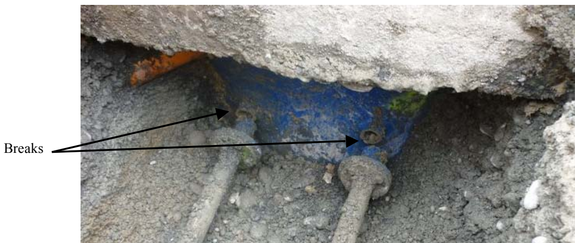
Photograph 13: Birchgrove Pump Station, Christchurch (PS97): Discharge pipes broke during 22 February 2011 earthquake at fibreglass spool just outside pump station wall.
