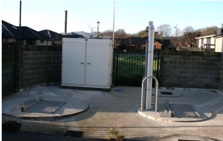
Photograph 12: Linden Grove Pump Station, Christchurch (PS96). No damage during earthquakes of 2010 and 2011. Pump station and valve chamber are close, and tied together with concrete slab.
