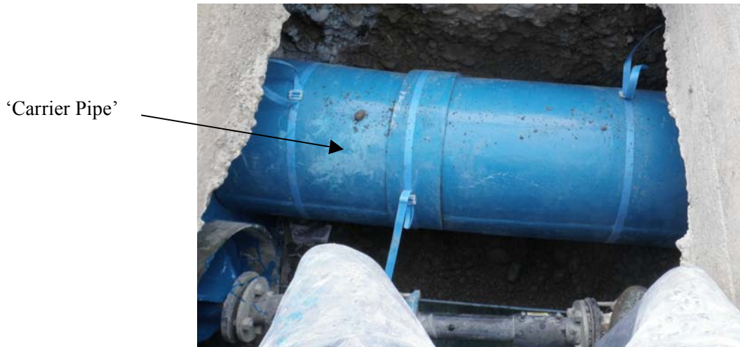
Photograph 14: Birchgrove Pump Station, Christchurch (PS97) Earthquake Damage Repairs: (1) Fibreglass nozzles strengthened, HDPE pipe used, and 'Carrier Pipes' being installed to provide room for movement.
