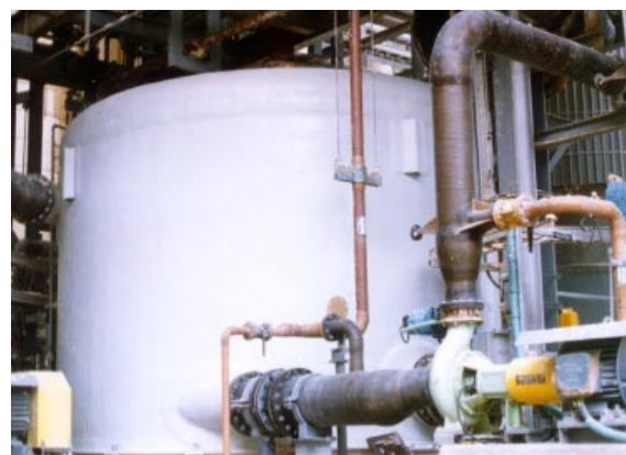
Fibreglass tank at pulp and paper mill handling corrosive washer filtrate liquor.
