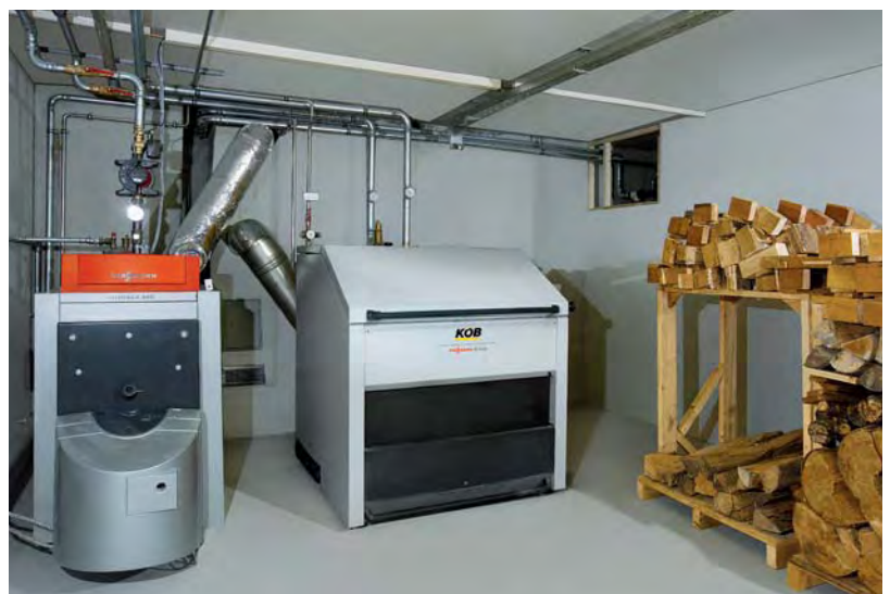
Pyromat ECO log boiler with adjacent Vitoplex 300 low temperature oil boiler
