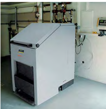
Pyromat ECO log boiler heats a two-family home in Niederbipp (Switzerland)
