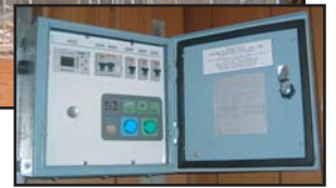
Bushlight Energy Meter
