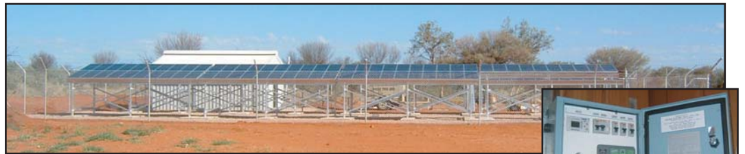
Bushlight Community RE system at Akanta
