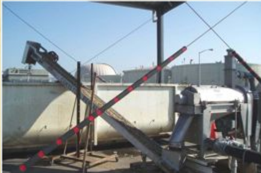
Photograph from EBMUD Odor Control Master Plan, CH2M Hill (2009)
