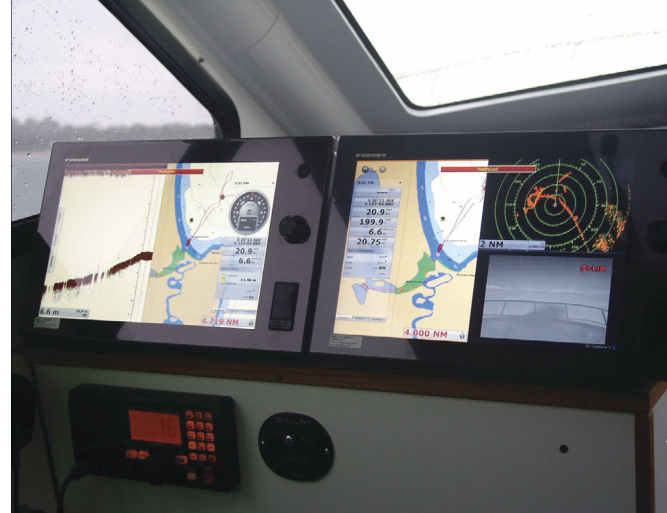
Left and Above: Well known Furuno identity - not to say guru - Shane Beardmore working with the incredibly powerful Furuno Nav-Net multi-function system installed in the new Noosa Cat 3500. Shane is seen here explaining to Mandurah’s Barry Walton all the functions and potential of this incredible system - whilst Mandurah VMR Commodore Ian Walton watches on.
