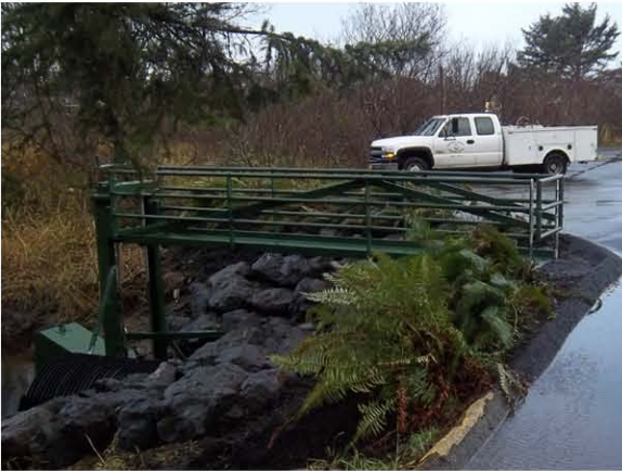
Walkway to MTR unit so that the adjustment handle can be reached to set MTR to the interior water level that the tidegate will close at.
