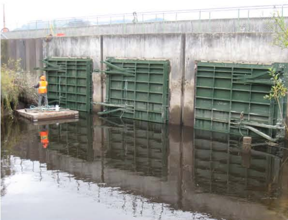
These massive NSRG 9 x 11 tidegates are mounted to aluminum frames which are anchored to the concrete wall. All three gates are operated by a single MTR system.
