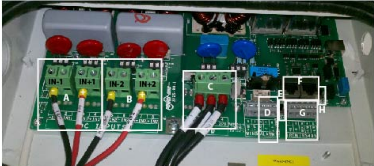
Figure 2:10 Main Inverter Connection Board
