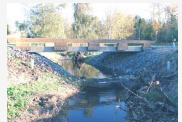
The bridge seen here, installed by NSEA in 2014, improves the opportunity of returning salmon to navigate upstream toward Lake Terrell. No longer is this section of the creek difficult for salmon to pass.
