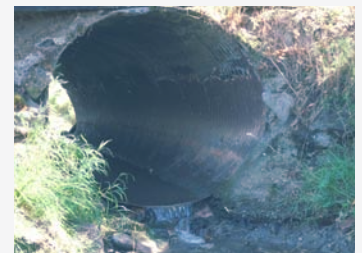
Replacing fish passage barriers, like the culvert (above) with bridges (below) first takes a willing landowner, in this case Myrna Louveau.
