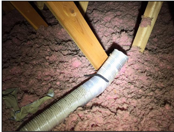
29. Not well secured
