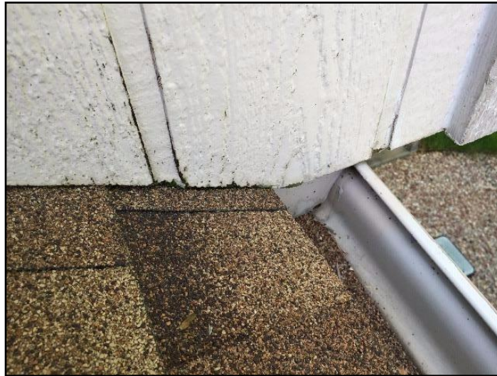
4. Siding not cut back
