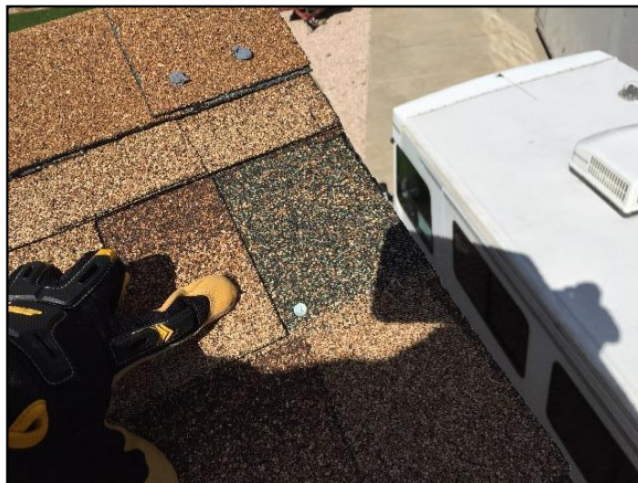
3. Missing, loose or torn
