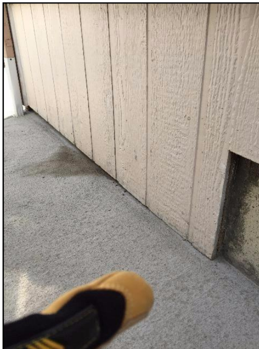
10. Too close to grade
