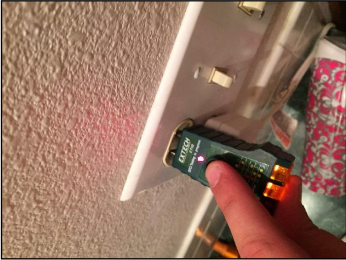
17. No GFI (Ground Fault Interrupter)
