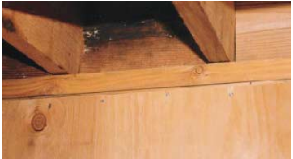
Figure 4. This shear plywood should have extended to the top of the double top plate — a mistake that can be remedied with the addition of metal connectors across the two plates.
