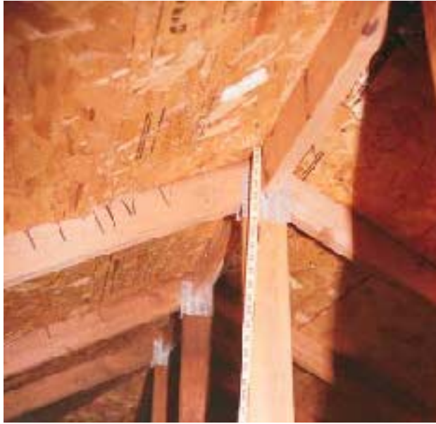
Figure 1. Nails that miss the truss — a result of sloppy work with a pneumatic nailer — void the strength of the roof diaphragm.
