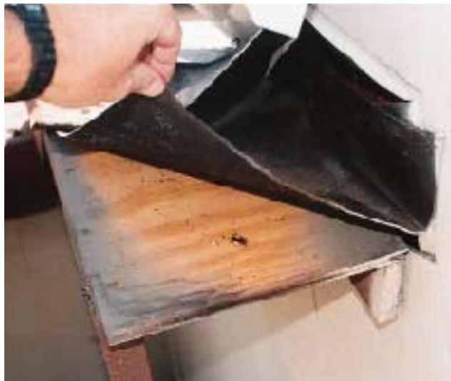
Figure 7. Instead of folding down over the edge, the felt paper on this rake overhang was cut flush with the top of the sheathing, allowing rain water to wet the surface of the roof deck.
