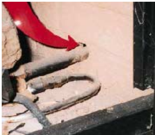
Figure 23. The pipe penetration into a gas fireplace must be properly sealed with a firestop material — a defect that's easy to spot and easy to fix with fireproof grout.
