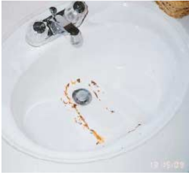
Figure 18. The chipped enamel in this cheap lavatory sink is the kind of defect that will send condo or tract homeowners ballistic — especially when they see it in every home on the block.
