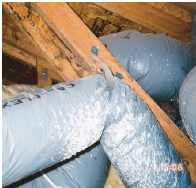
Figure 20. A pinched duct can result in uneven temperatures. It's easy to fix if it's accessible, but easier still to avoid.
