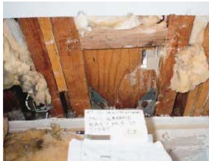
Figure 5. These shear wall hold-downs are too close together, making the shear wall practically useless in resisting overturning forces.
