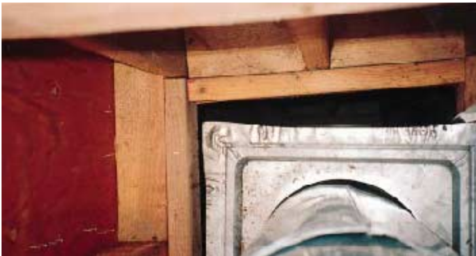
Figure 22. Firestops are an important safety requirement. Unfortunately, if a gap is missed by the inspector, all too often it will be permanently concealed from view.
