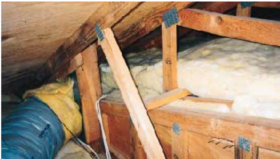
Figure 2. The plywood on this interior shear wall should have been carried all the way to the roof diaphragm.
