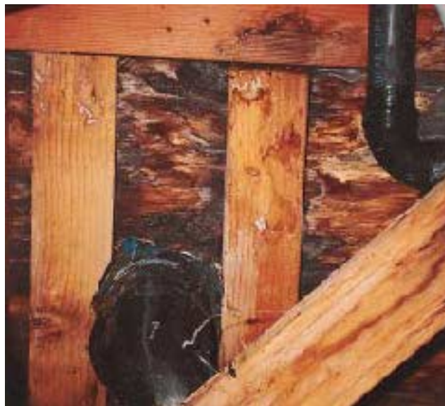
Figure 17. If hidden by finish surfaces, a leaky toilet connection can go undetected until structural decay sets in.
