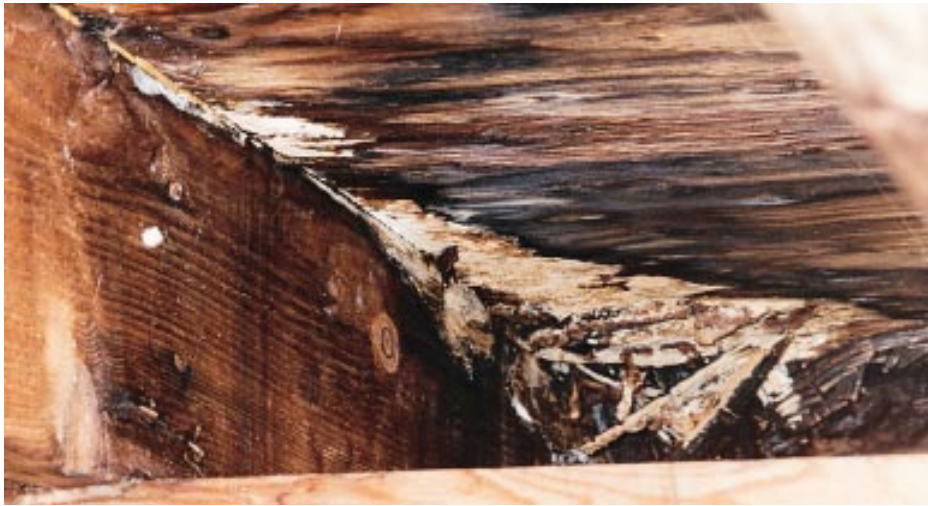
Figure 15. Because waterproof decks are difficult to detail properly, rotting substructure is a common defect.
