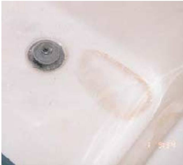
Figure 19. Ponding in the bottom of a tub unit — the result of an out-of-level installation — is not structurally serious but is obvious to any homeowner.
