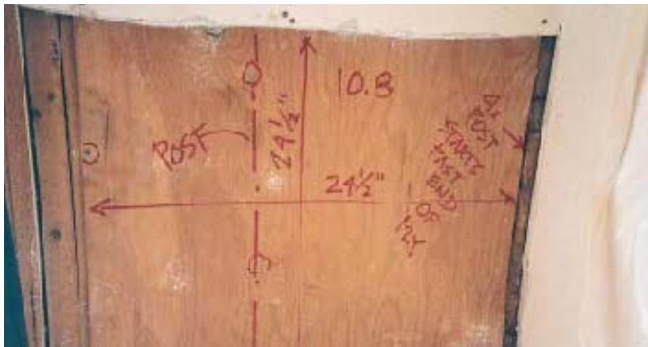
Figure 3. This shear plywood falls short of the shear wall posts on the right and left, and is attached with too few nails.
