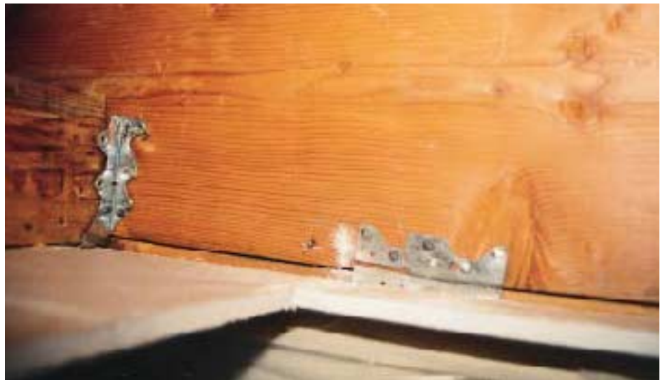
Figure 6. An inspection made through a hole cut in the ceiling reveals that the joist hanger at left is bent and missing nails.
