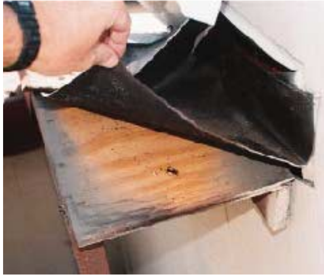
Figure 7. Instead of folding down over the edge, the felt paper on this rake overhang was cut flush with the top of the sheathing, allowing rain water to wet the surface of the roof deck.
