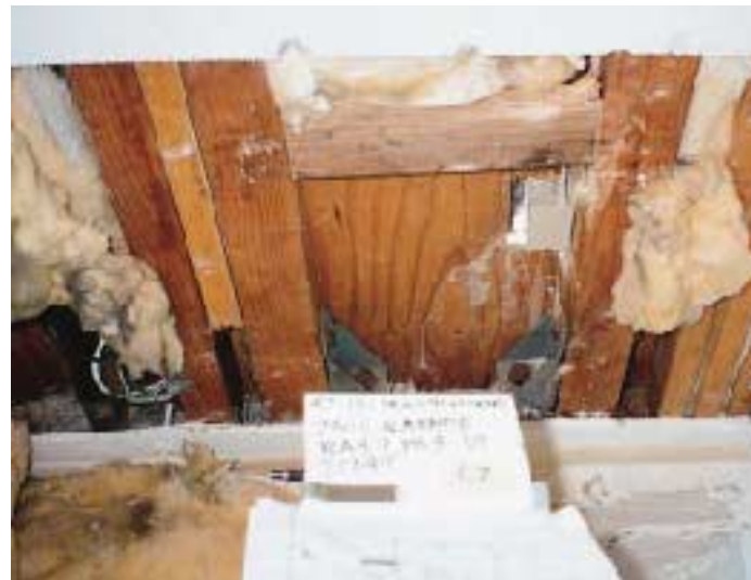
Figure 5. These shear wall hold-downs are too close together, making the shear wall practically useless in resisting overturning forces.
