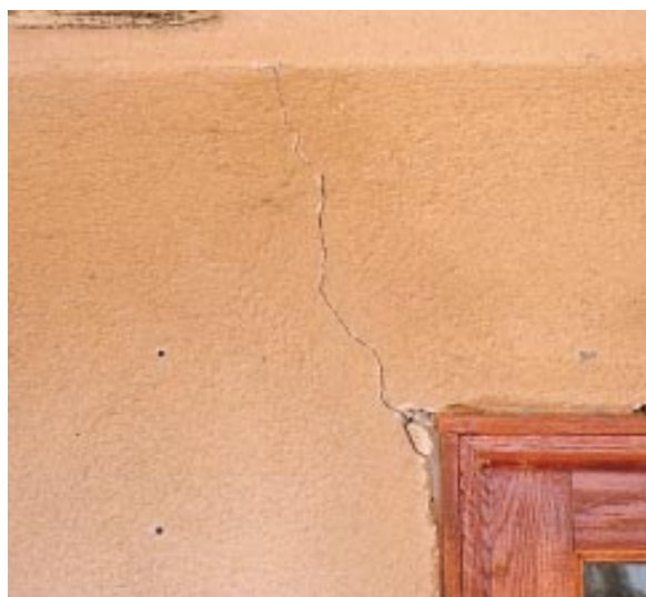
Figure 14. Stucco cracking is one of the most common customer complaints. Tight surface cracks are normal in stucco and can usually be repaired. With quality workmanship, larger cracks can be avoided.
