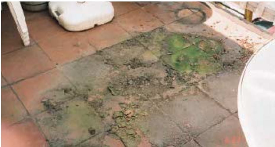
Figure 16. Besides ruining the finish surface, ponding on waterproof decks also leads to deterioration of the framing below.
