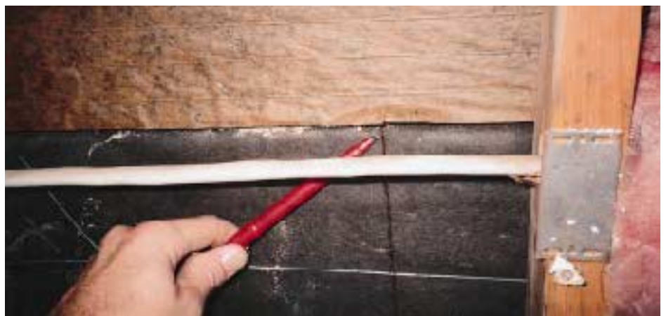
Figure 9. The building paper below a window must be tucked below the flashing paper — a detail often botched, as in the top photo. Above is a reverse lap seen from the inside of the wall cavity.
