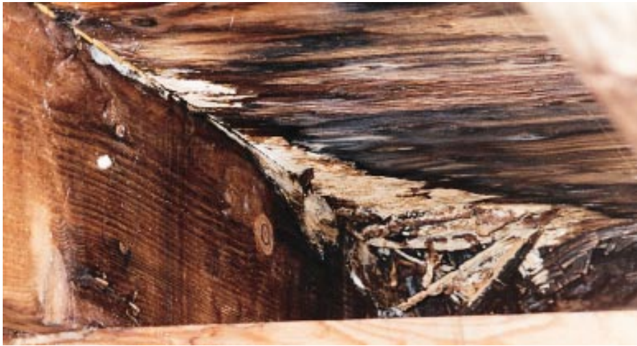
Figure 15. Because waterproof decks are difficult to detail properly, rotting substructure is a common defect.
