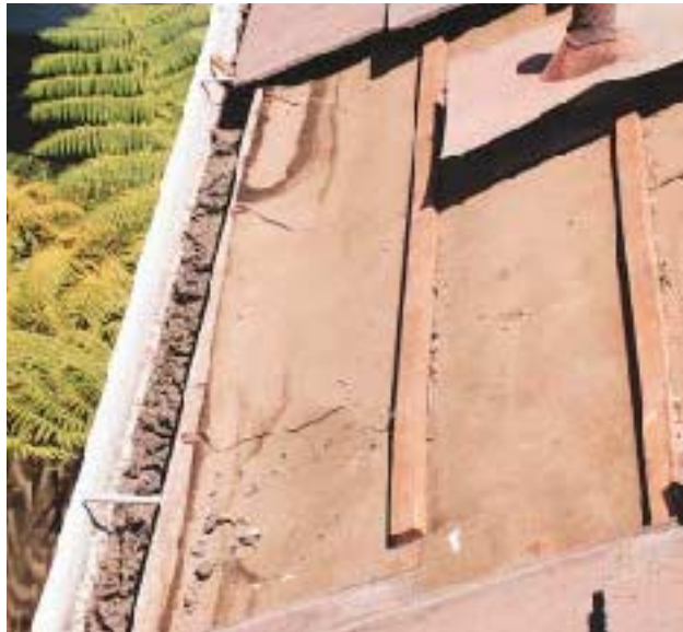
Figure 8. A raised fascia board (illustration) requires a heavy metal flashing or cant strip to ensure that runoff passes over the edge. Otherwise, water will pond, as in the photo, resulting in leaks and rot in the eaves.
