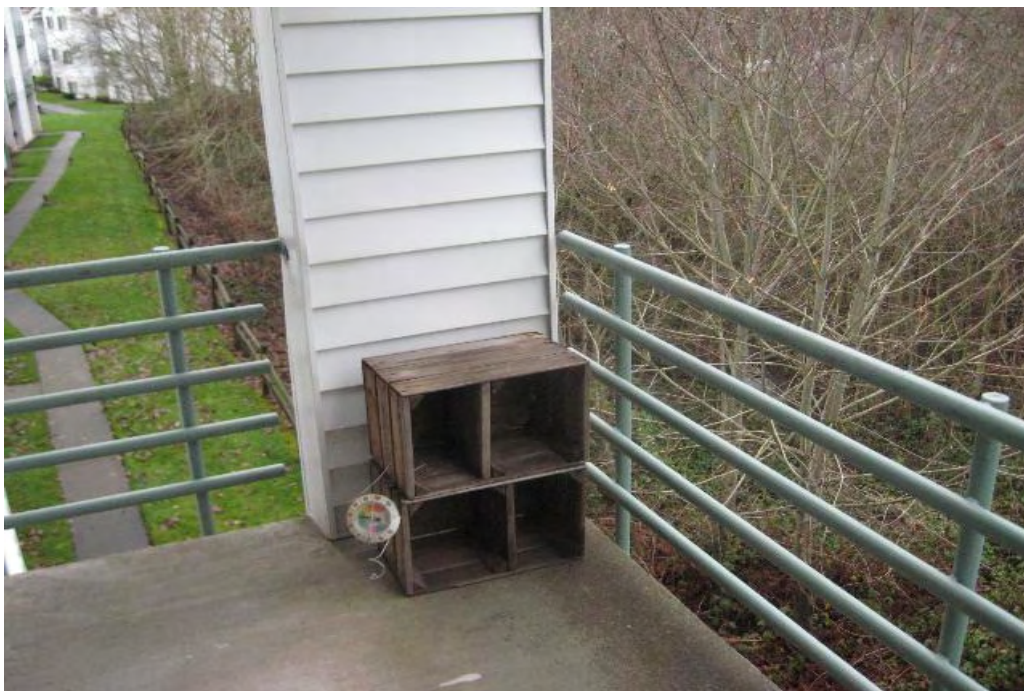
SM 01.043 Unit #49; Back elevation; Deck railing. Side guardrail at left, main guardrail at right. Note attachment to wall at right side of left guardrail.
