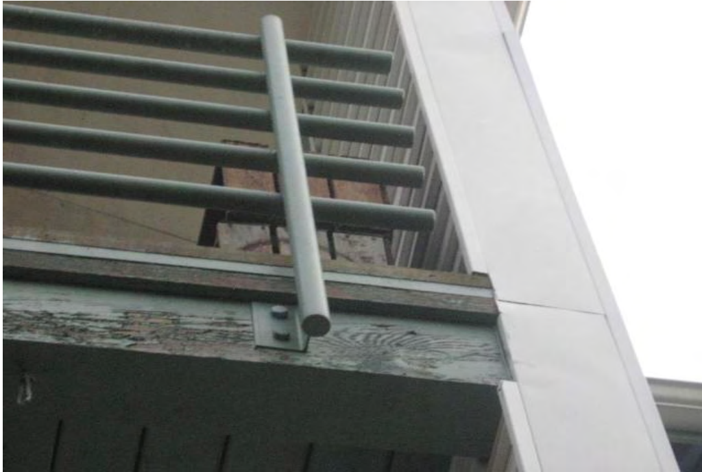
SM 01.038 Unit #49; Back elevation; Deck. Main guardrail fastened to beam with large lag bolts.
