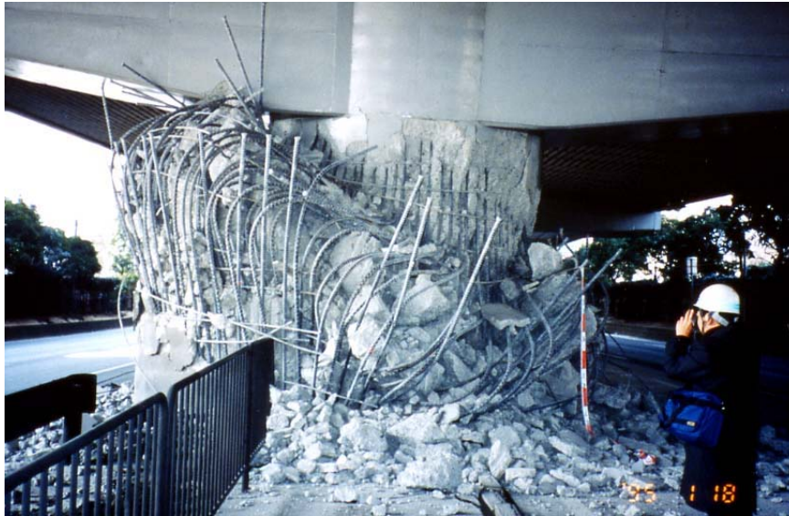
Damage in this column is unacceptable
