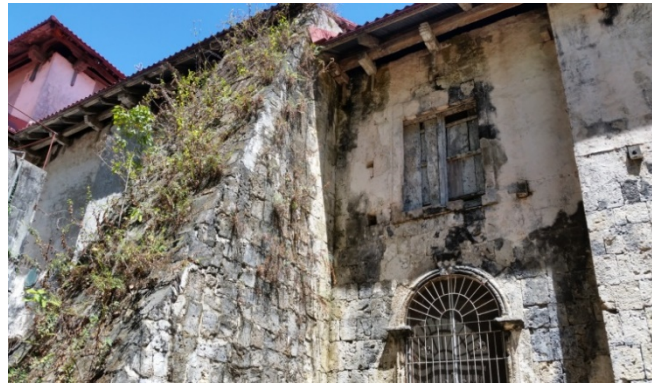
Cracked walls above arched doorway needs repair and strengthening.
