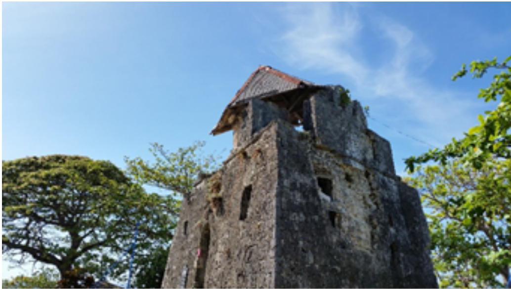
Close up of Tower showing extent of delamination
