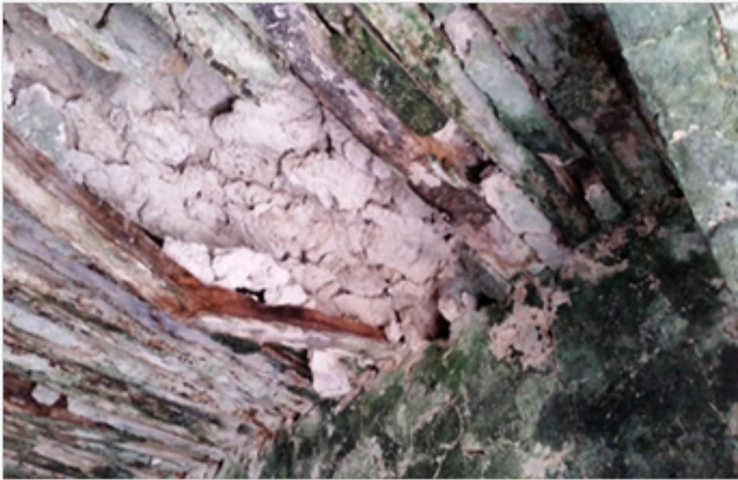
Damaged or missing Timbers require replacement
