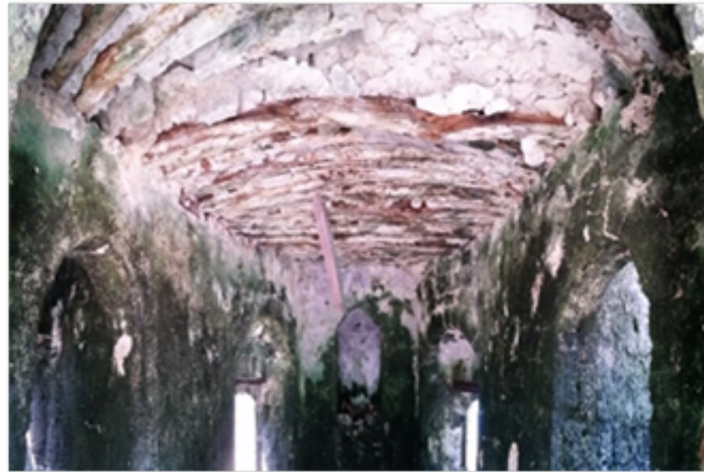
View of interior Floor Support show damaged
