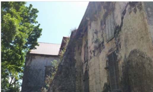
Exterior wall cracks with growth of moss requires repair, strengthening and sealing.
