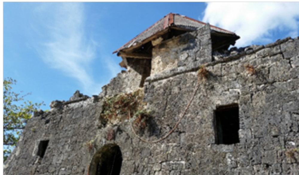
Top portion of Tower showing extent of damage
