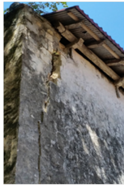
Walls separation at corners needs repair to prevent accidents.
