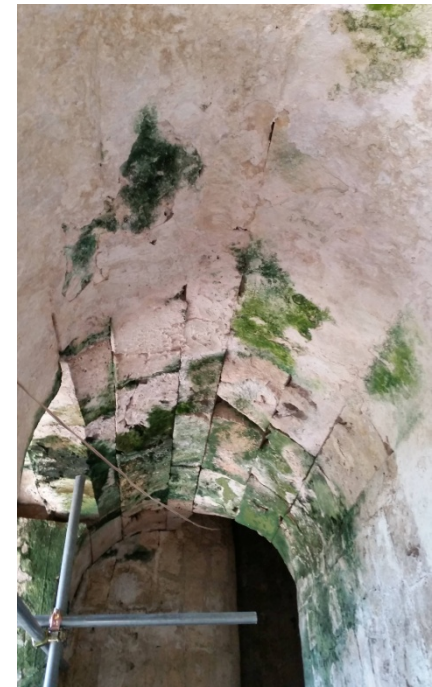
Arch shows movement of Voussoirs. Repair required.
