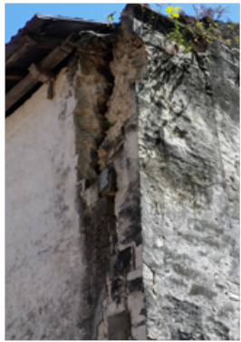
Large delamination of wall at corner requires anchoring and repair to prevent falling hazard
