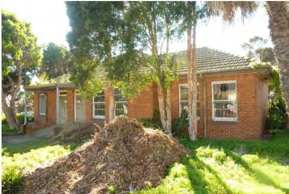
Figure 4 North Western elevation of Building 1. This portion of the building, near the Middle Head Road frontage is to be retained within the overall scheme.
