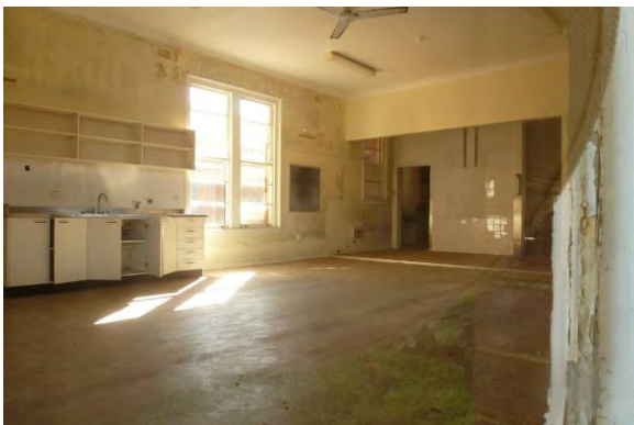
Figure 6 Large internal room in Building 3, illustrating the fine quality of the internal light emanating from the large side windows.
