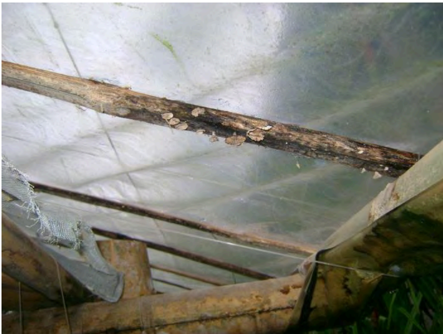
Photo 11 Damage to bamboo from water leaking
