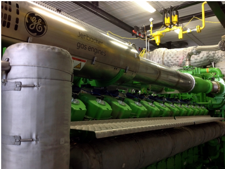
Figure 45. CHP system in California: A Jenbacher J624 two-staged turbocharged natural gas engine. Credit: © GE
