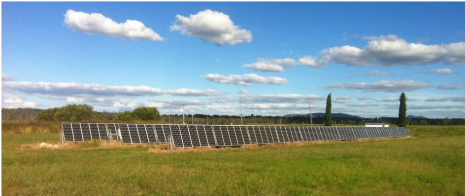
Figure 19: 30kW solar PV plant at Glen Cairn dam
