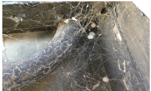
The retreat of a reback living inside an electrical box, complete with egg sacs.
