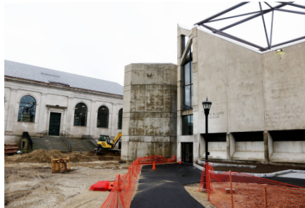
Construction sites surround the new entrance to Love Gym. By Gavin Hickey/The Exonian
