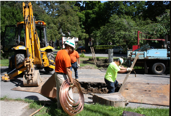
City workers install the new spigot at Morrison Park. It will now be much easier to water the flowers and plants in the park. Photograph courtesy of Jim Hondorf.
