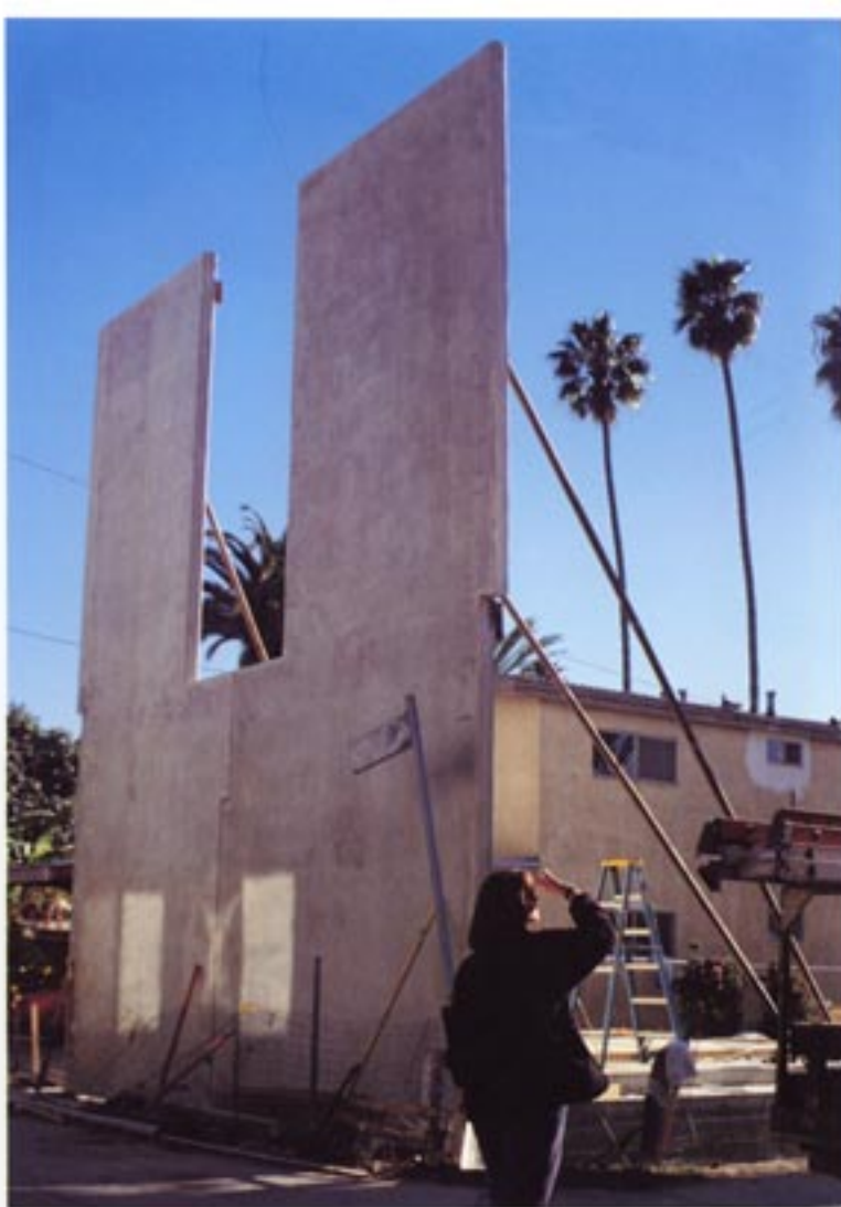
Hertz's design consisted of fourteen six-inch-thick tilt-up concrete panels facing each other along the longitudinal edges of the site, which composed an elongated interior space. The structure was erected in just ten hours.
