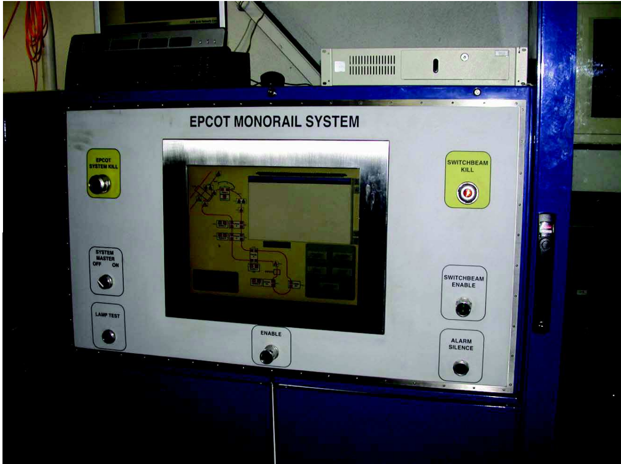
Figure 4. Power Distribution and Monitor System switch panel for controlling switch-beams 8 and 9.
