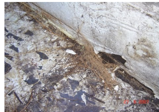
Roots tearing membrane
