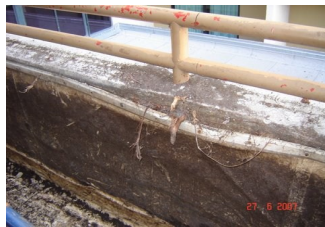
Roots growing behind membrane
