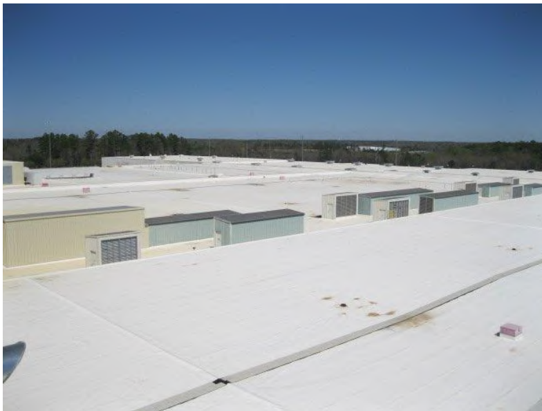
This is a partial overall view of one area of the main roof.
