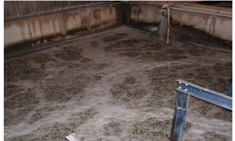
Aerated Primary Reactor
