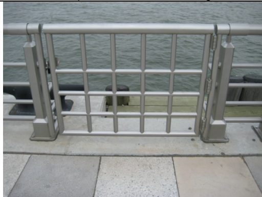
Gangway gate aligns with piling and cleat so gate cannot be used for gangway
