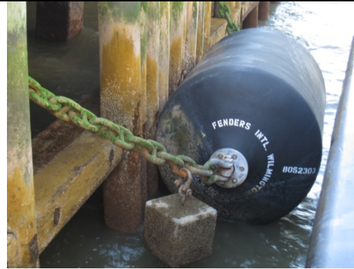
5' wide Yokohama fender, scaled to larger ships than most intended under “historic ship” RFP designation, so custom gangways or rigs are needed to span them adding more cost.
