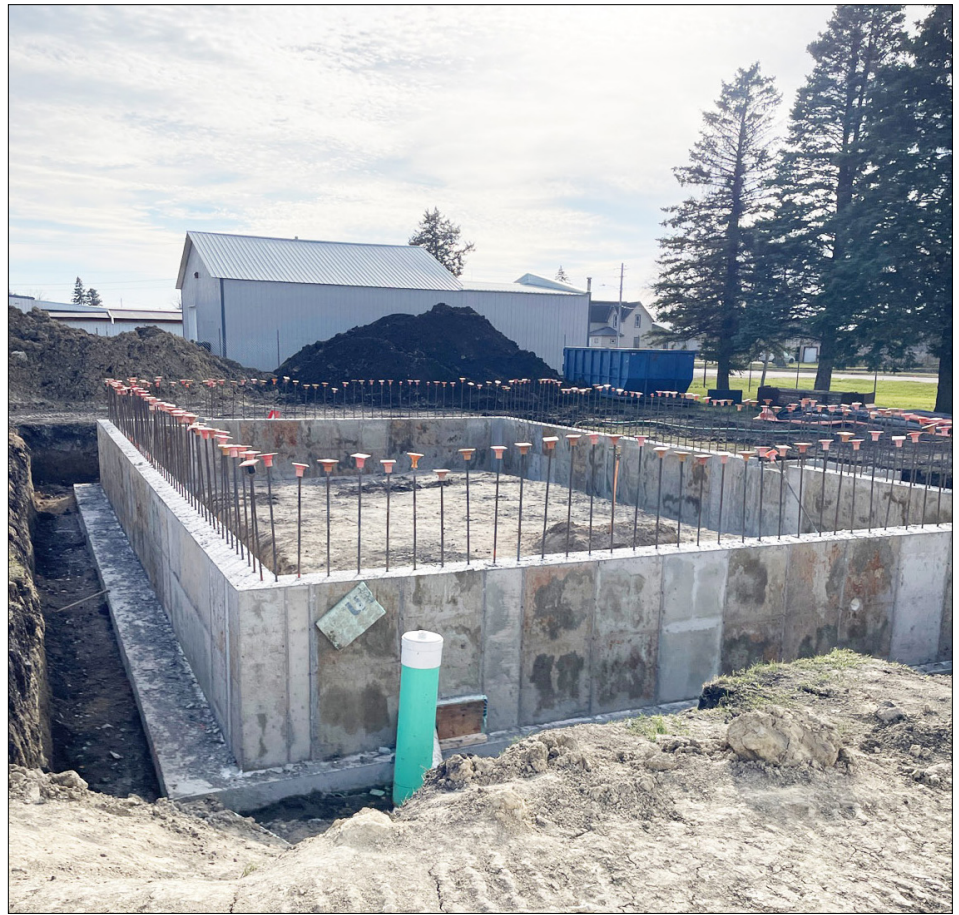
Completion of the Madelia storm shelter was originally estimated for late summer 2024, but warmer winter conditions allowed contractors to work through the winter and move up the completion date to June.
