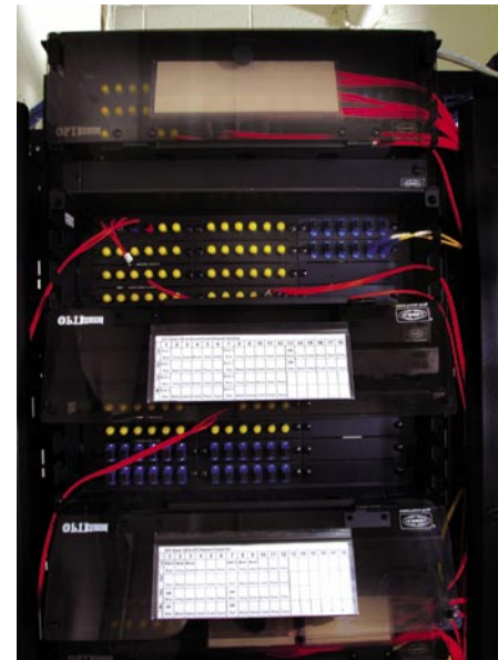
Front view of local and wide area fiber patch panels in the communications room of the Central Station building
