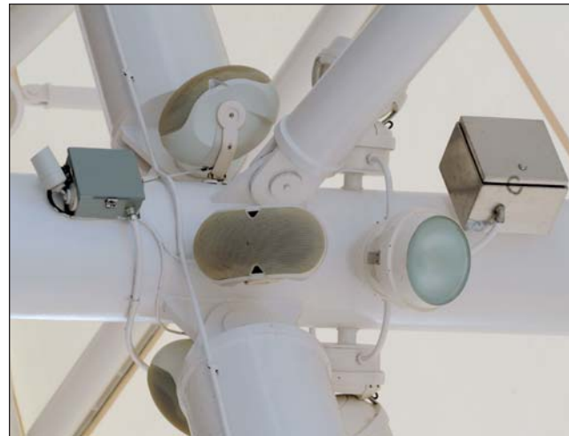
Above, infrastructure is an important element of the security and communications design at the Grand Rapids bus station. Columns on the Central Station platform hold lighting, audio and security video cameras with the latter attached to a pullbox allowing all cables to route through the structural column.
