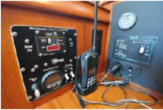
> nav station electronics
