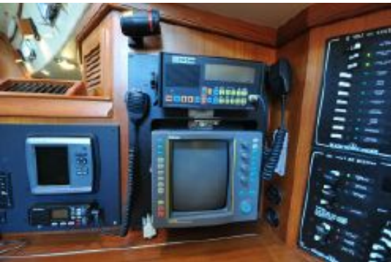
> nav station electronics
