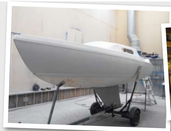
The topsides were primed and painted with three coats of International Perfection Undercoat...
