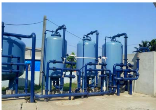
91,500 m3/hr Arsenic & Iron Removal System in Bazitpur Village, Barasat, North 24 Parganas
