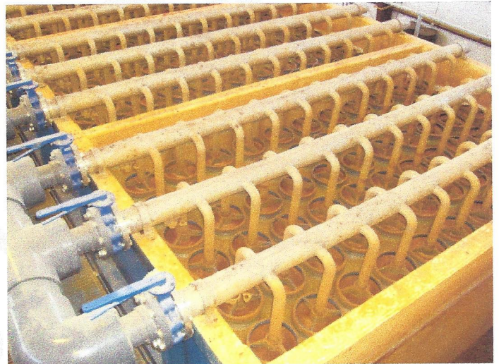
Figure 4. UF membranes in holding tank.
