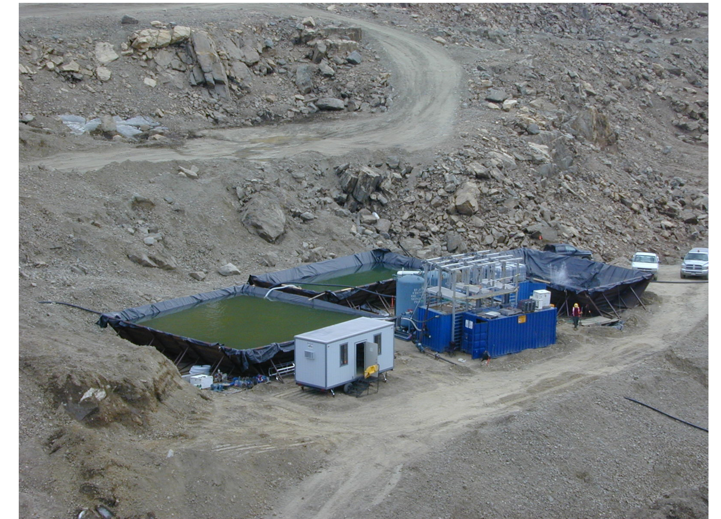
Figure 1: The above picture was taken of an electrocoagulation system that was being used in a dam resurfacing project in Colorado.
