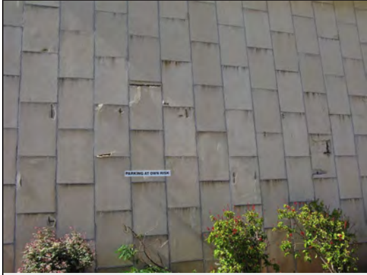
Figure 14. Spalling concrete wall
