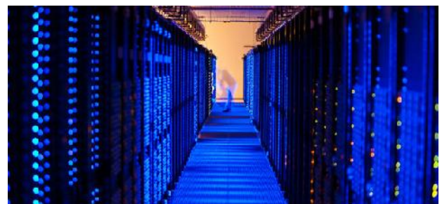
Amazon AWS Datacenter. Source: New York Times
