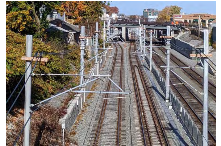
Figure 52: Overhead Contact System Overview - Poles and Guy Wires Suspend the Contact Wire above Each Track (MBTA Green Line Extension; Somerville, MA).
