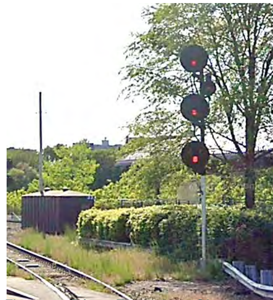
Figure 51. Example Signal at Interlocking Where a Branch Line Joins the Mainline (Worcester Mainline Merge in Framingham)
