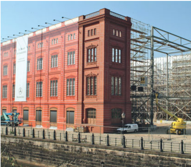
Karl Friedrich Schinkel, Bauakademie, Berlin, 1836, destroyed 1961/62 Following the reconstruction of a small model facade in 2001, the erection of a complete demonstration facade in 2004 gave a new impetus to discussion about the reconstruction of the Bauakademie.
