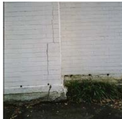
Fig. 8 Cracked foundation on home due to the shrinking and swelling of Houston Black clay it was built upon. Credit: Clay Robinson
