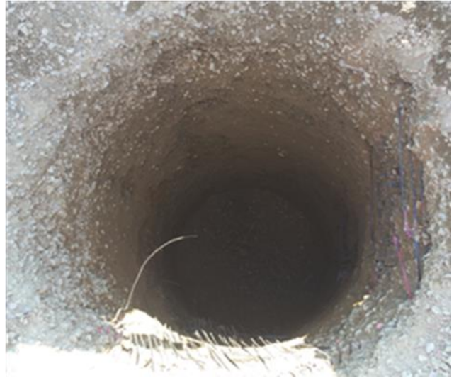
Fig. 7. Geogrid Sheared and Supporting the Drilled Hole
