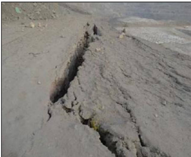
Fig. 4. Longitudinal tension cracks related to toppling failure mechanisms along sub-vertical joint structures exposed in the underlying bench.
