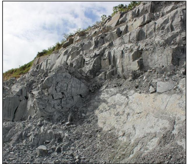
Fig. 5. Back-break of benches due high fragmentation from poor blasting as well as unfavourably orientated joint structures.
