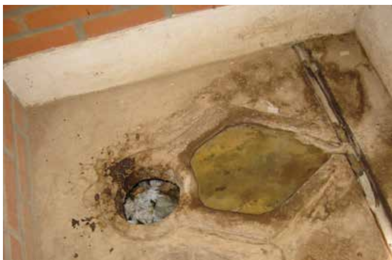
The drain in this UNICEF-built urine diverting dry toilet was blocked due to improper use and lack of maintenance.
