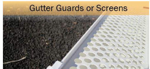
Figure 37. Rain gutters should have screens to keep leaf debris from accumulating. Maintain gutters to keep them clear and clean.
