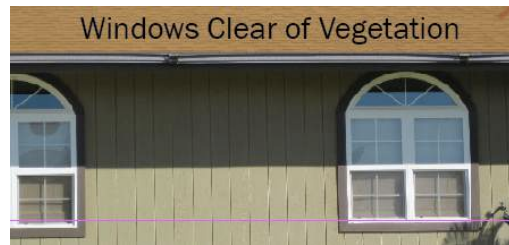
Figure 35. Keep windows free of vegetation to reduce likelihood of heat-caused breakage that lets embers into your home.
