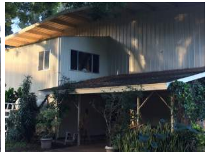
Seabury Hall, example of debris on roof
