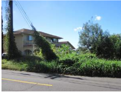
Hazardous vegetation growing on powerline
