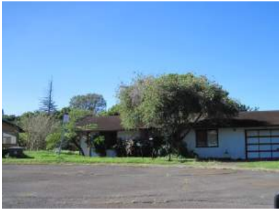
Example of home with vegetation overgrowing roofs and walls
